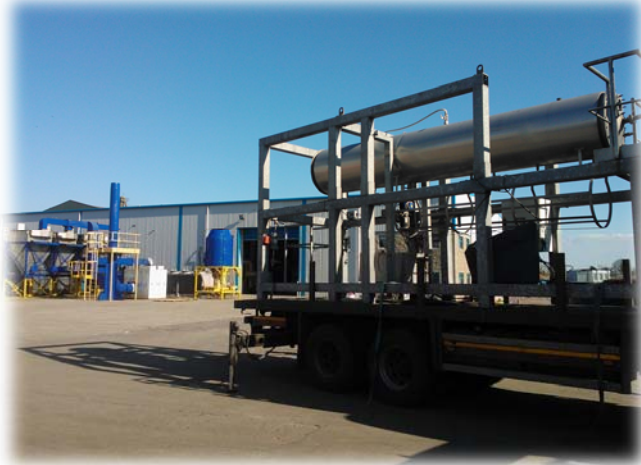
Photo on left shows pre-commercial scale wastewater treatment technology (on truck-bed) developed by TCBB & NUI Galway with NVP Energy—produces biogas; also, Premier Green Energy's advanced pyrolysis technology (located on the site of the former Thurles sugar factory) is in the background
